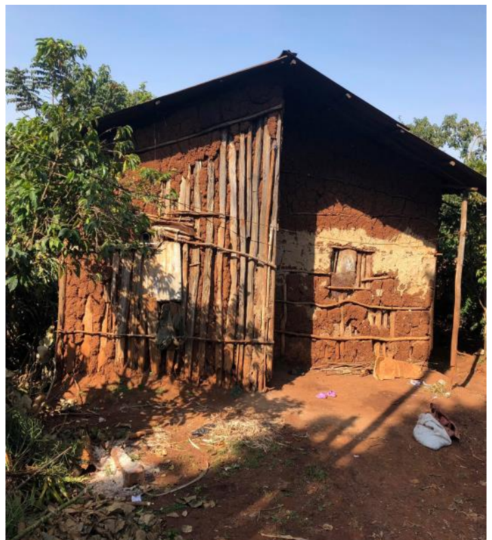
Above: One of the homes in urgent need of repair.
